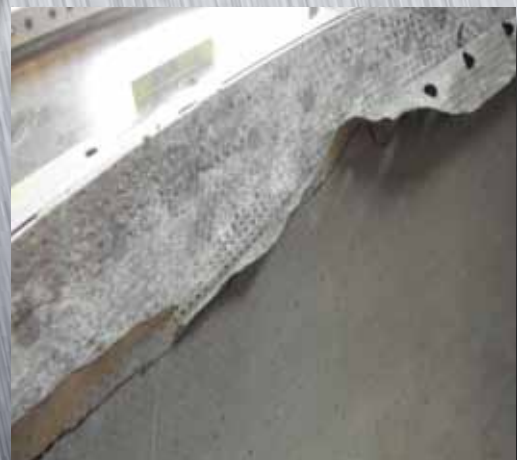
Delamination of the Composite Structure
